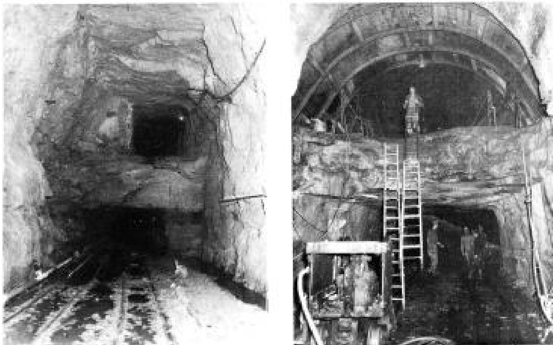
Photo 3.1 - Views showing methods adopted in tunnelling work near Martin Place station in 1954 (source PTC of NSW archives)
